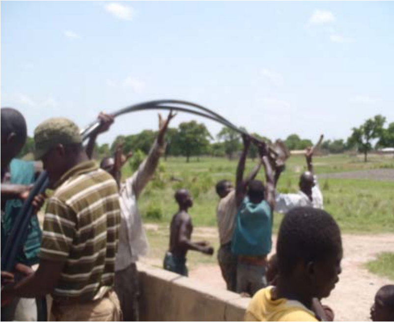
Project in process and community members assisting the LWI Burkina Faso team with the water project.
